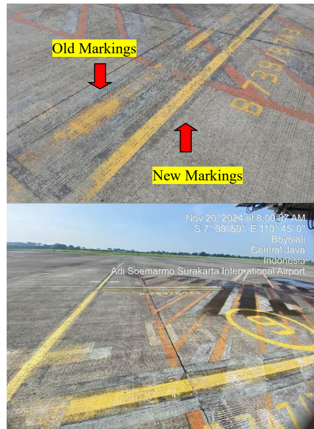
Figure 3. Condition of Parking Stand 6 Apron Markings
